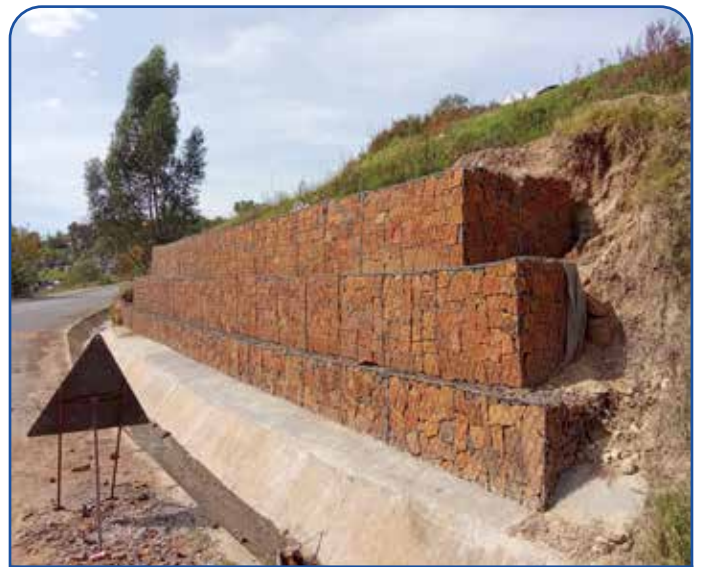
Periodic maintenance of C- Point to Moshoeshoe Airport Roads intersection and C-point bypass
