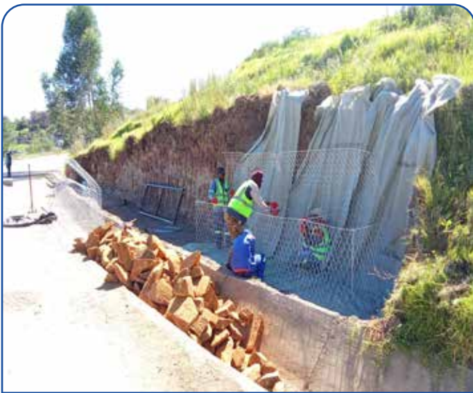
Periodic maintenance of C- Point to Moshoeshoe Airport Roads intersection and C-point bypass
