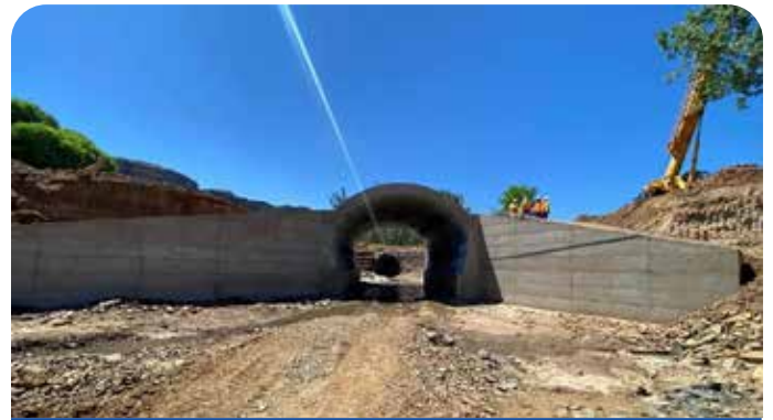
Emergency repair of of Peka major culvert crossing Sekutukutu river on the A1 to B11 road
