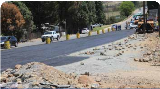
Repairs and re-sealing of A3 Road from Masianokeng to St. Michael's and the construction of Masianokeng intersection
