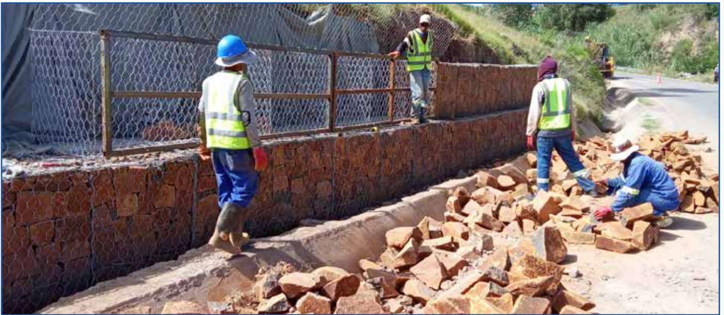
Periodic maintenance of C- Point to Moshoeshoe Airport Roads intersection and C-point bypass
