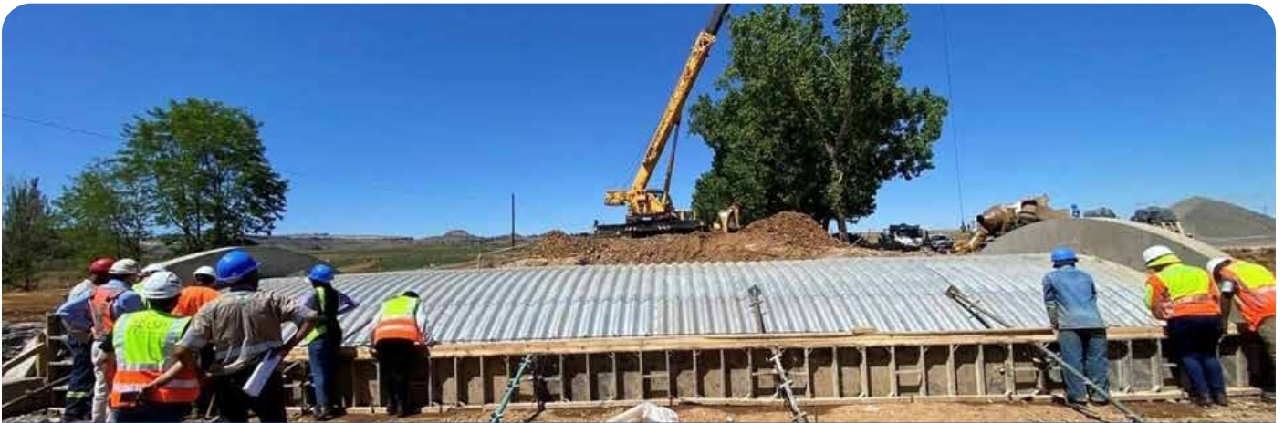
Emergency repair of of Peka major culvert crossing Sekutukutu river on the A1 to B11 road
