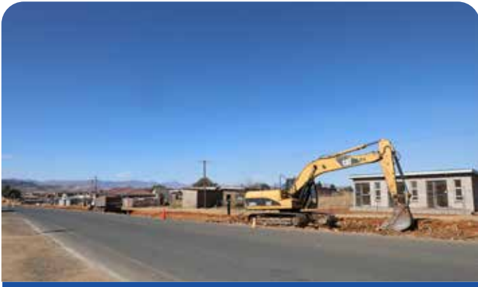
Repairs and re-sealing of A3 Road from Masianokeng to St. Michael's and the construction of Masianokeng intersection
