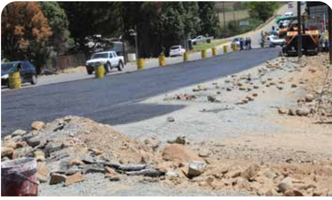
Repairs and re-sealing of A3 Road from Masianokeng to St. Michael's and the construction of Masianokeng intersection
