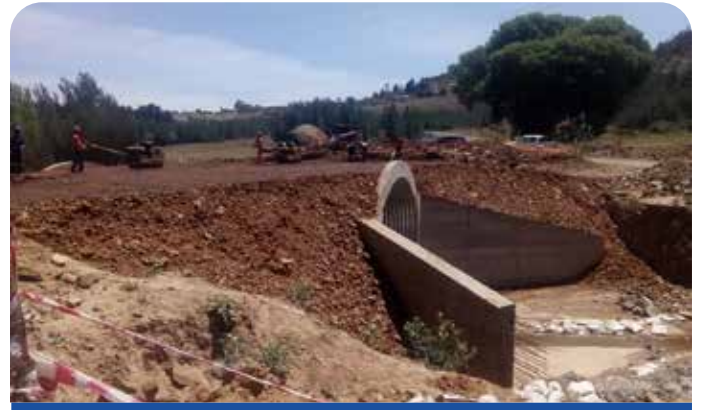
Emergency repair of of Peka major culvert crossing Sekutukutu river on the A1 to B11 road
