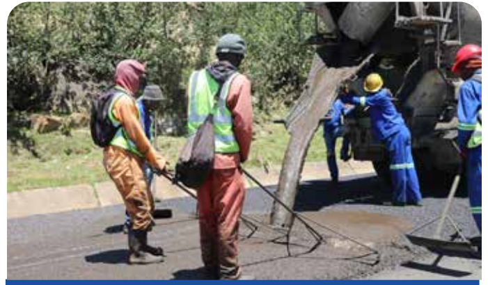
Repairs and re-sealing of A3 Road from Masianokeng to St. Michael's and the construction of Masianokeng intersection
