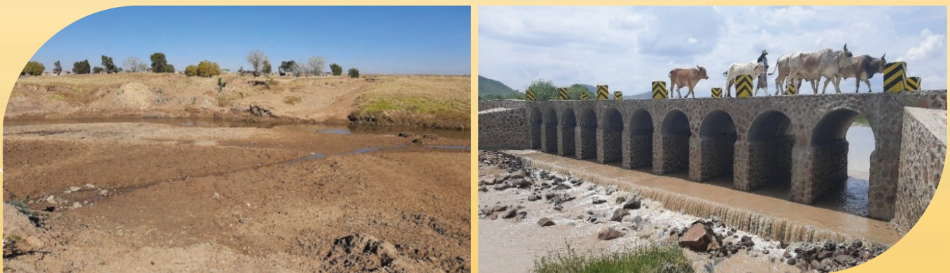
Pic Collage 1: Periodic Maintenance of Bongalla to Maoela Gravel Road, construction of Mini Bridge sponsored by Road Fund and implemented by the Ministry of Local Government and Chieftainship. Picture providing the before and after conditions.
