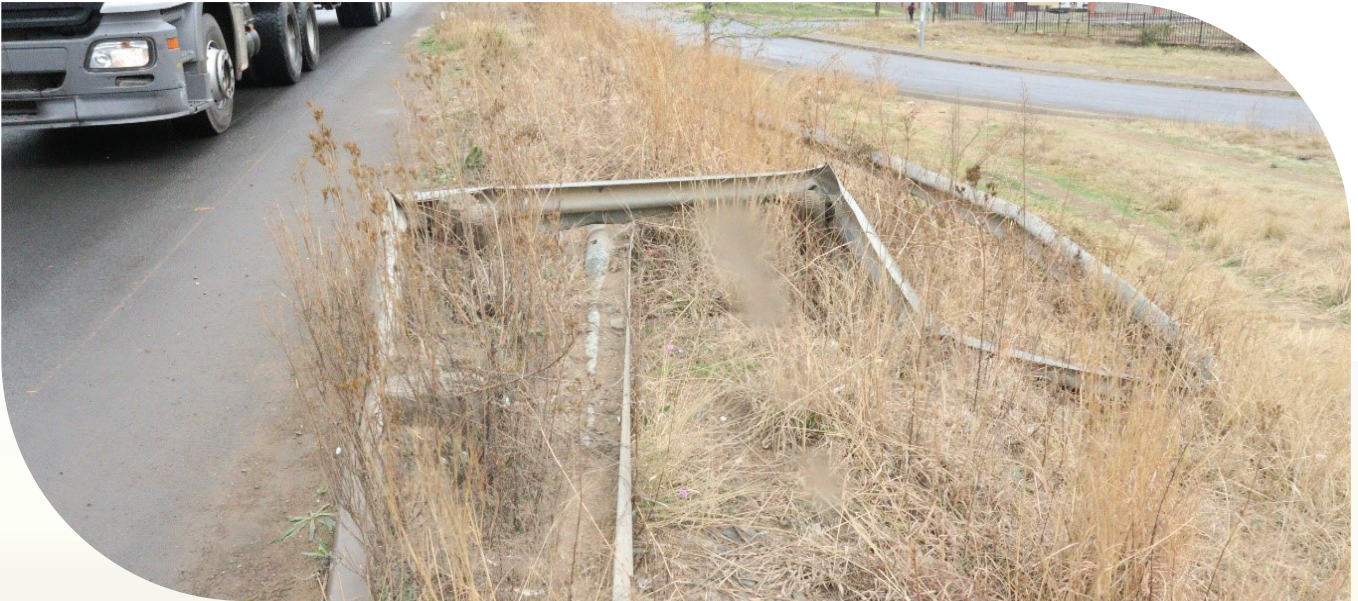
Pic 3: Guardrails Damaged by vehicles have been identified as part of the Audit
